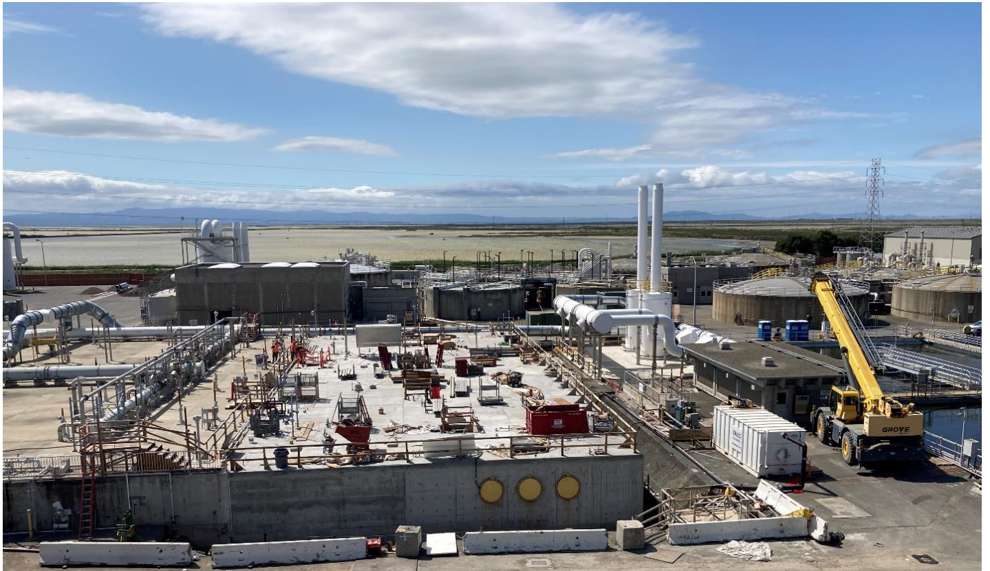
ETSU Aeration Basin Project Cover Picture: Motor Control Panels at New Aeration Basins
