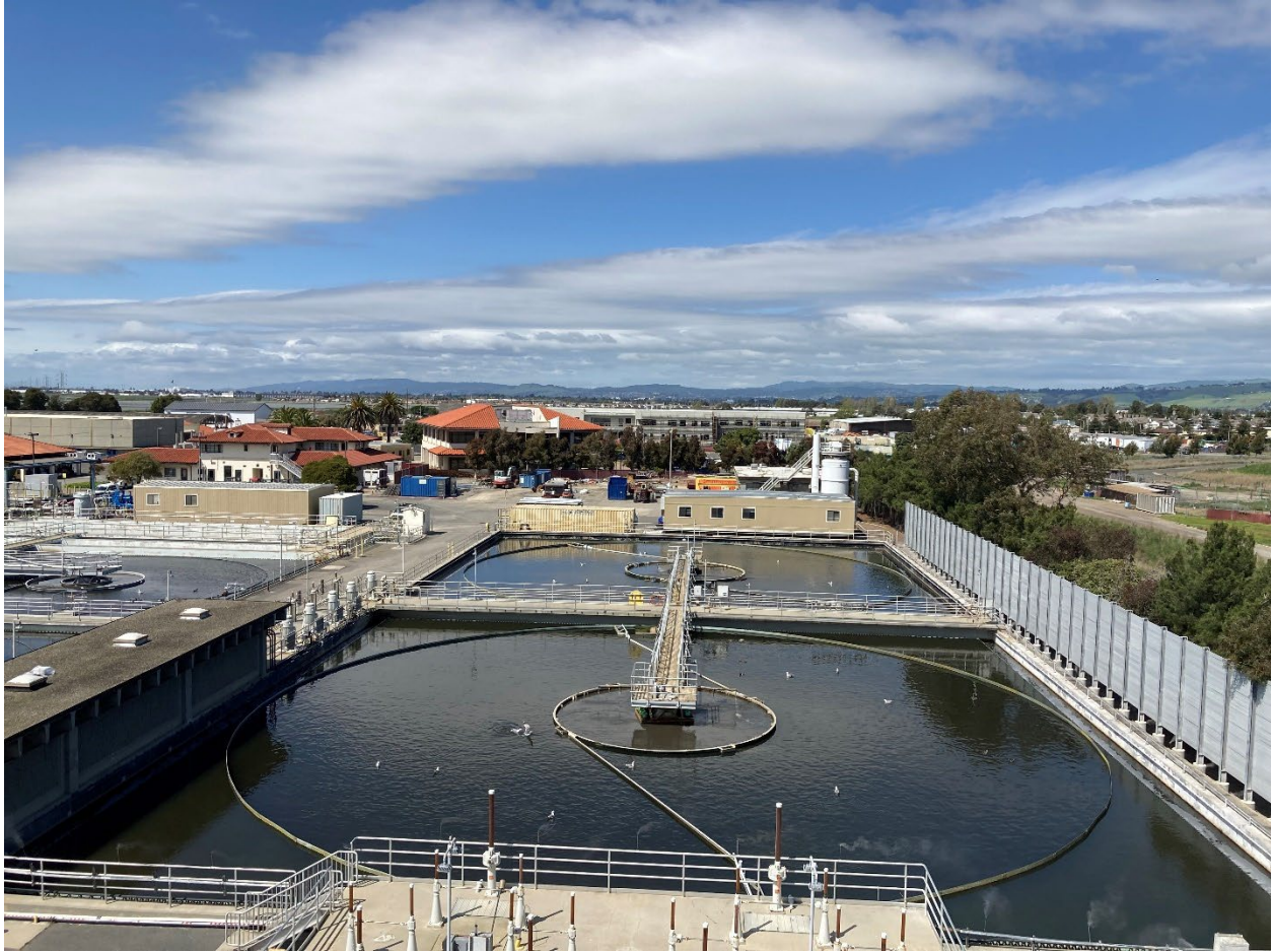
View Northward over the Secondary Clarifiers
