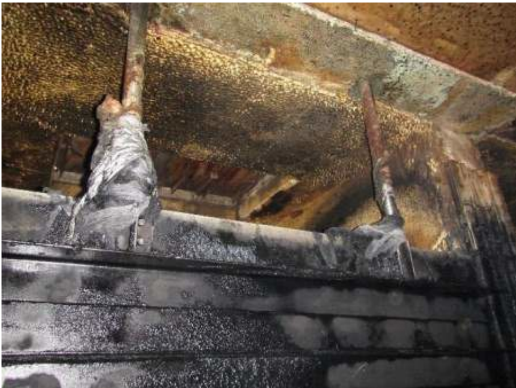
Figure 6 – View toward ceiling and typical weir gate that controls flows from CB1 main compartment to a primary clarifier distribution box
