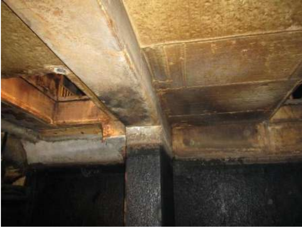
Figure 5 – PVC liner at the northeast ceiling with exposed concrete beam
