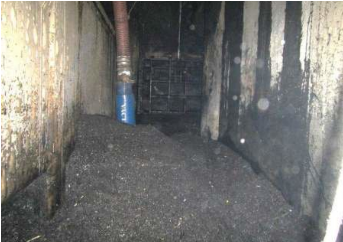
Figure 4 – View looking west at 60-inch dia. sluice gates and sediment buildup
