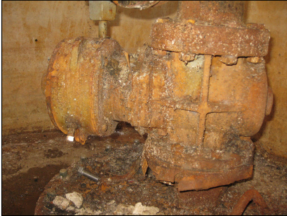
Figure 5 – Valve at Automall ARV Manhole
