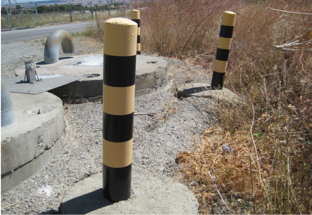
Figure 13 – Coyote Hills ARV Access Improvements, New Aggregate Access Pad Flush with Top of Manholes and New Retaining Wall
