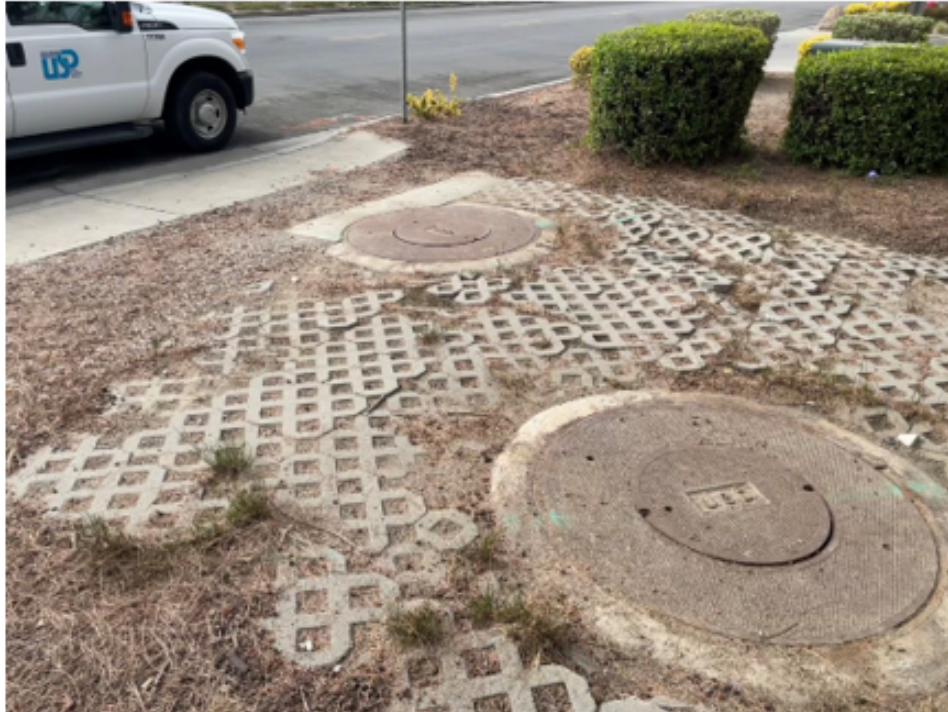
Figure 9 – Turf Block Pad at Morton Avenue Access Manholes
