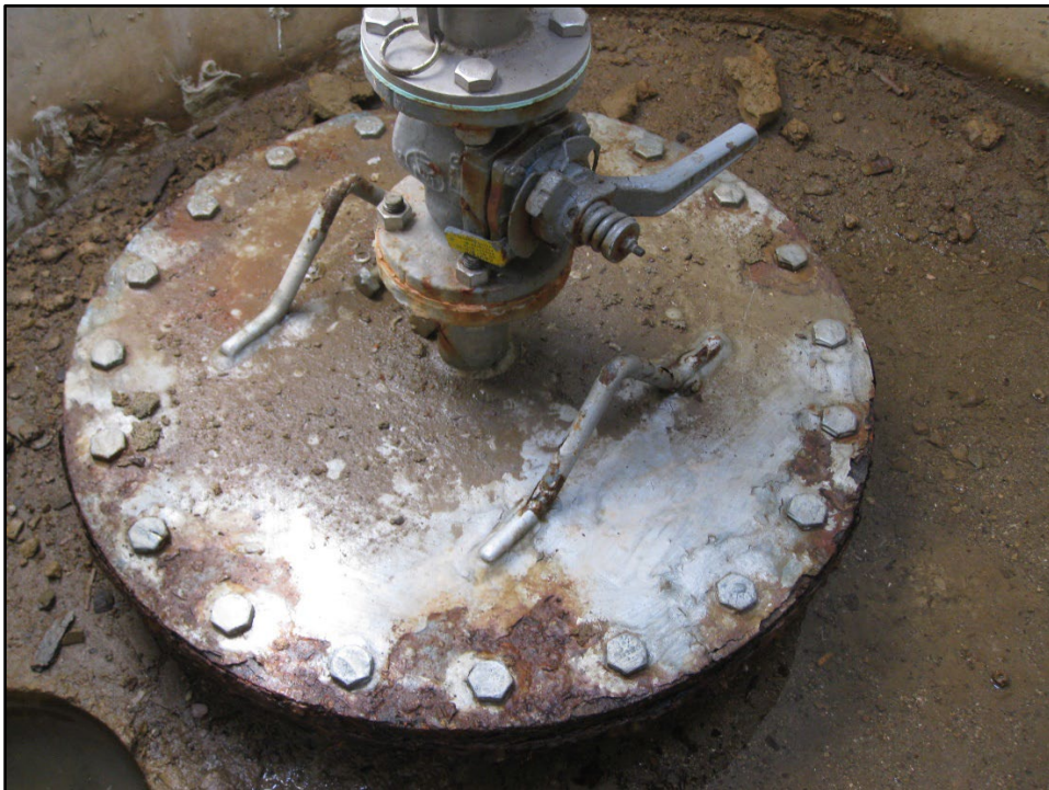
Figure 4 – Blind Flange at Boyce Road Access Manhole
