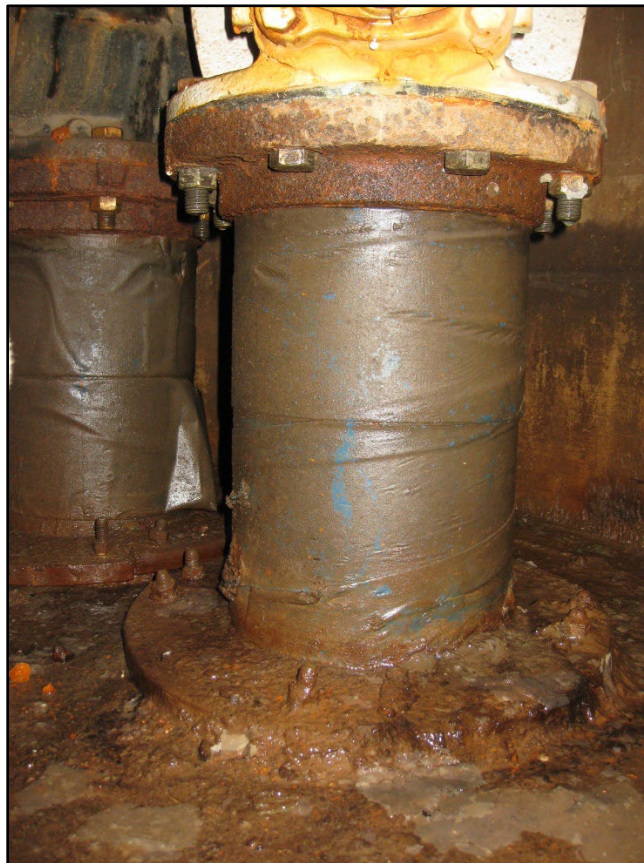
Figure 6 – Blowoff Tube at Cherry Street Blowoff Manhole
