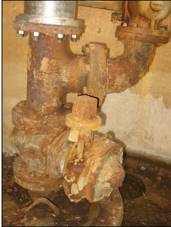
Figure 7 – ARV Piping at Cargill ARV Manhole
